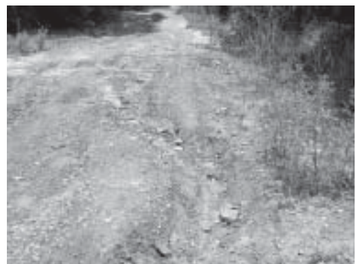
Figure 1-23 Be alert for signs that a road may be subject to washouts.
