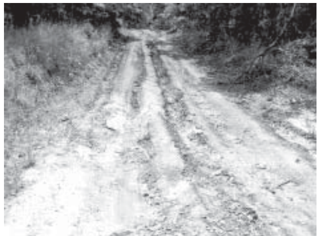
Figure 4-24 Ruts can easily develop over time in unpaved roads.
