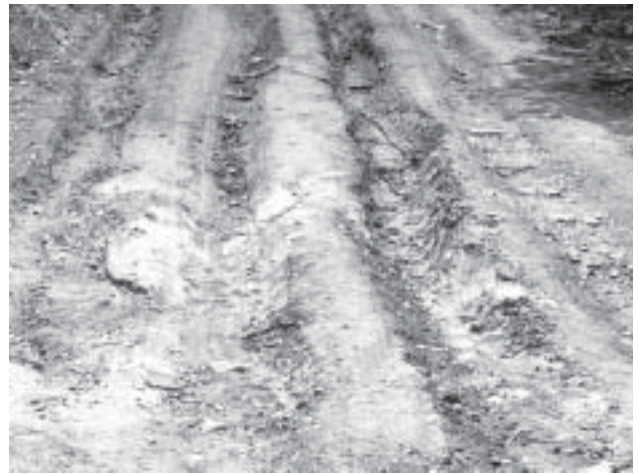
Figure 4-25 Be alert for serious deformities in unpaved roads.
