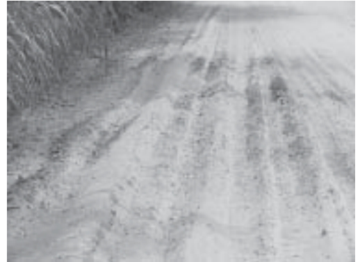
Figure 1-24 Unpaved roads may contain serious deformities.
